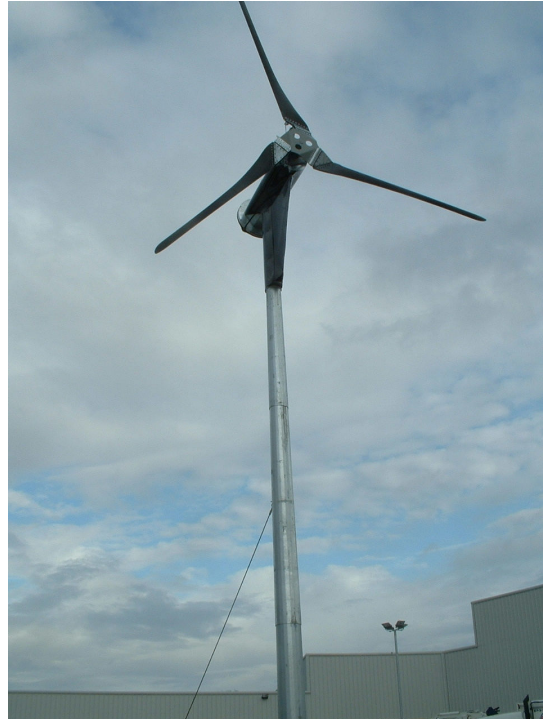
Wind Turbine eco Depot
