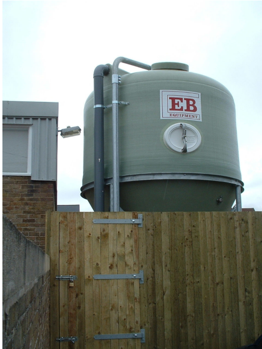
Wood pellet silo for Acomb Library
